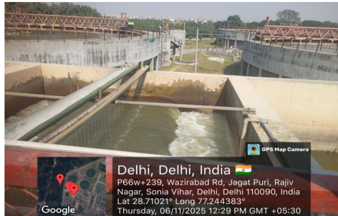
Pic. 1 Algae in settling tank
