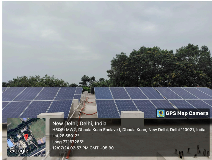
Solar panels in Science Block
