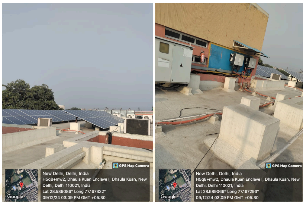
Solar panels installed at Art's block terrace
