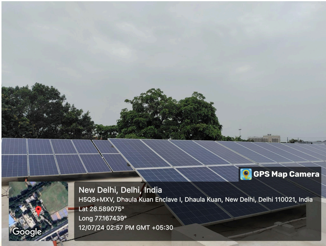
Solar panels in Science Block
