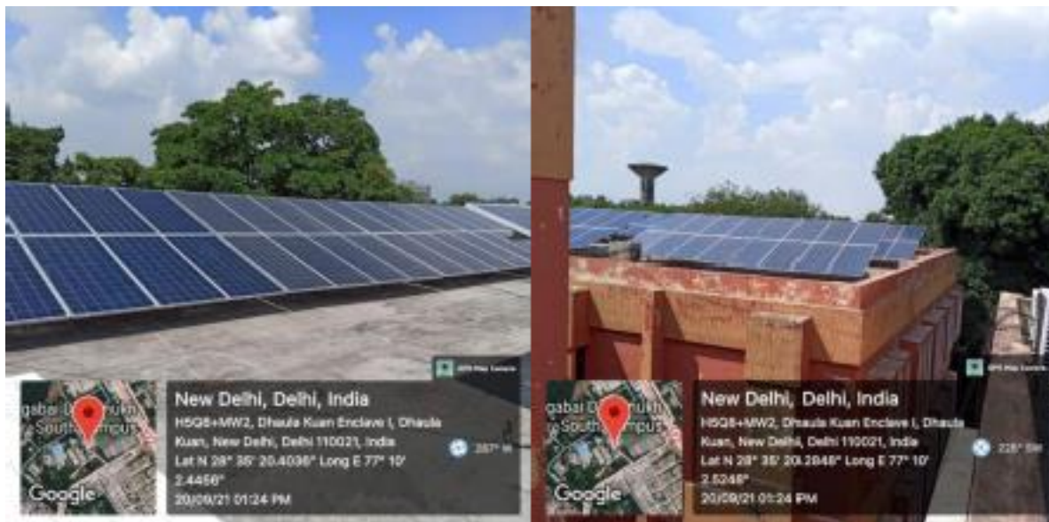
Solar panels installed at Art's block terrace
