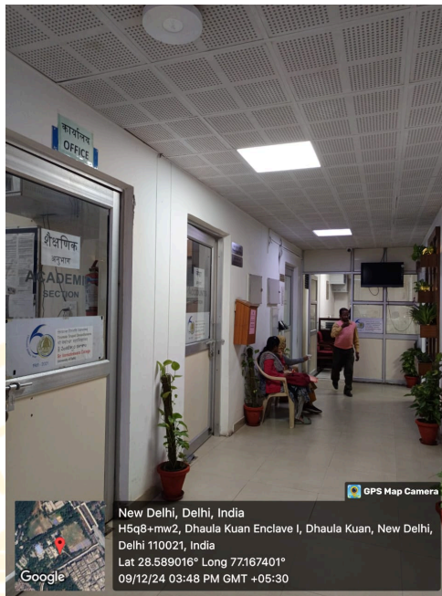
Administration section equipped with LED lights
