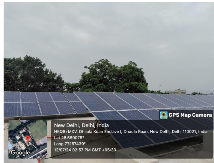
Solar panels in Science Block
