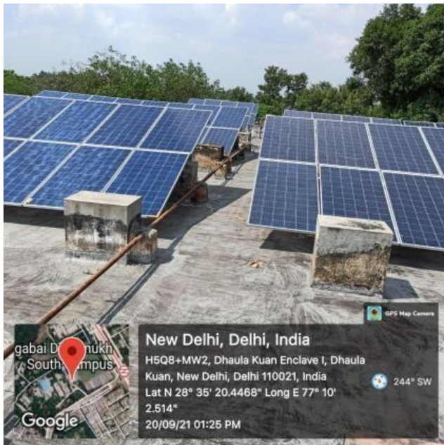
Solar panels in Arts Block
