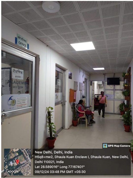
LED Lights installed in administrative block
