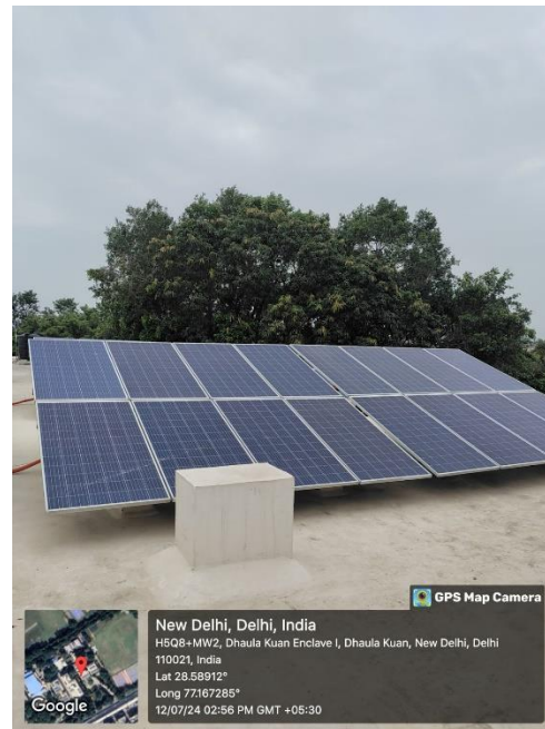
Solar panels installed at Hostel
