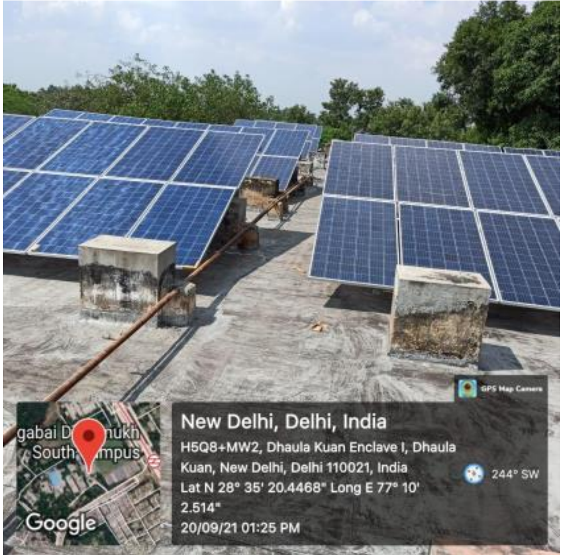
Solar panels installed at Art's block terrace
