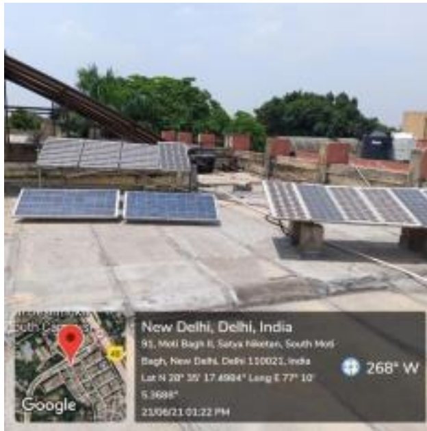
Solar panels in Science Block
